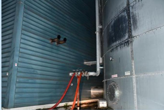
Figure 3.1 Replenishing the water supply via the connections provided for this purpose (Source: TBO VRR/VRZH)
