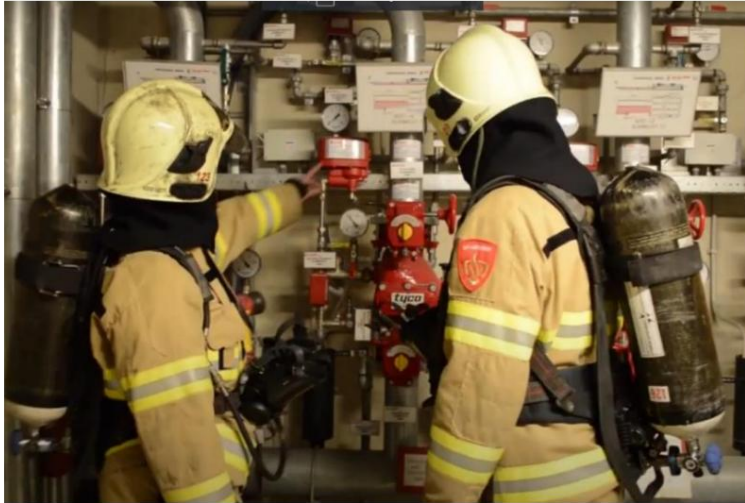
Figure 4.3 Firefighting team identifies the activated sprinkler section (Source: TBO VGGM).
