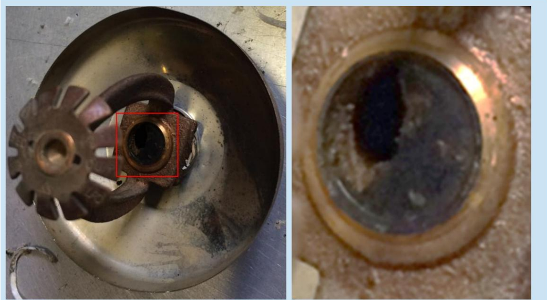
Figure 2.6 Contamination in the pipework leads to ineffective functioning of the sprinkler (Source: TBO VGGM)
