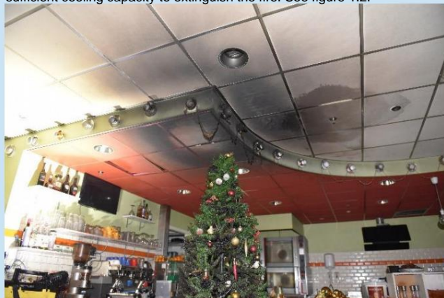
Figure 1.2 Activated sprinkler head near the seat of the fire (Source: TBO VGGM)
