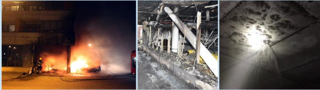
Figure 2.3 Images of the fire, the facade and the water yield from an activated sprinkler head (Source: TBO VGGM VRGZ)
