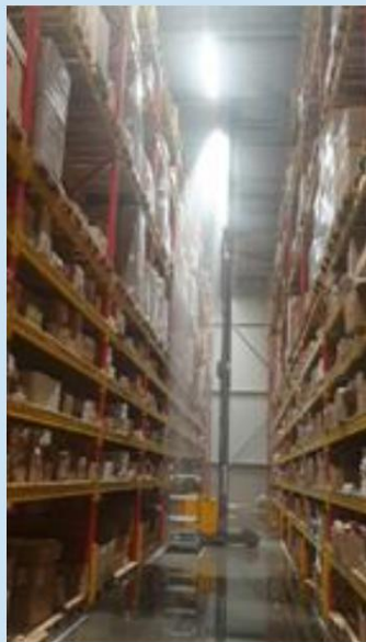
Figure 5.1 Activated sprinkler head in a warehouse (Source: VGGM)
