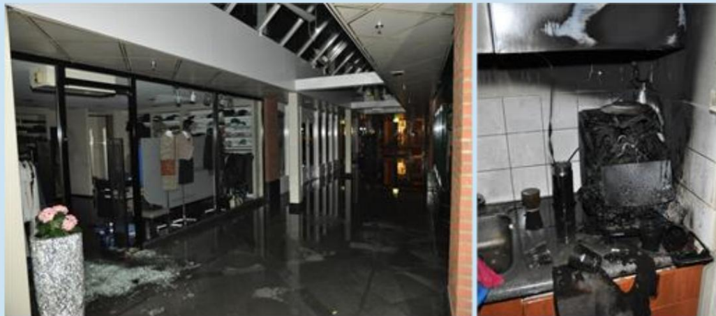
Figure 2.1 The shop on the left, the coffee machine that burned on the right (Source: TBO VGGM)
