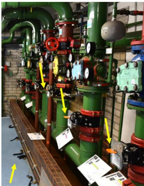
Figure 4.4 Closed valves of a sprinkler system; chains on the ground, the orange indicator on the valve is horizontal (closed) (Source: TBO VGGM)
